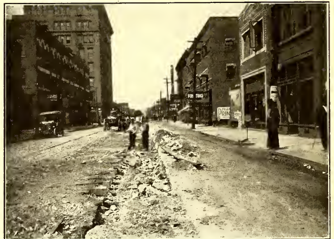
TAKING UP OLD CONCRETE IN DES MOINES (IOWA) BY PRYING AFTER DRILLING ROW OF HOLES 6 IN. APART WITH STEAM JACK HAMMER
